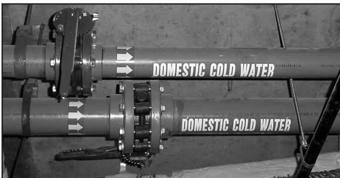
Butterfly valves installed with Corzan® pipe.
