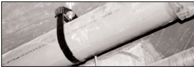
Typical pipe hangers.
